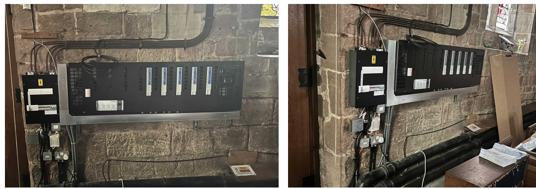
IMAGES OF LIGHTING CONTROL PANEL IN SITU
